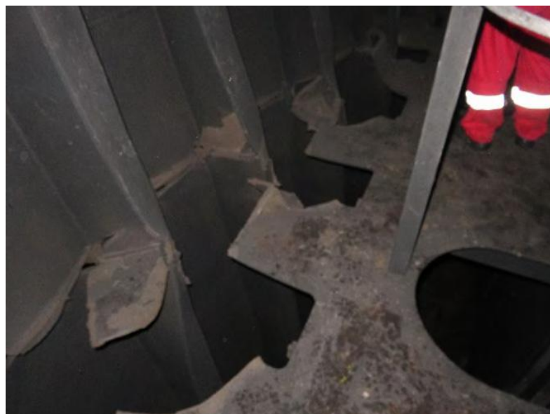
Fig. 2. Damage of bulkheads of residual tank m/t “Sri Asih”
